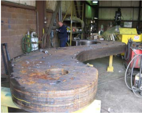
#1 Laminated hook plates are leveled, flame cut, predrilled and then tack welded together.
