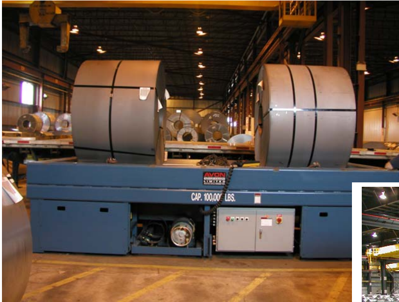
Propane powered transfer car for coil handling
